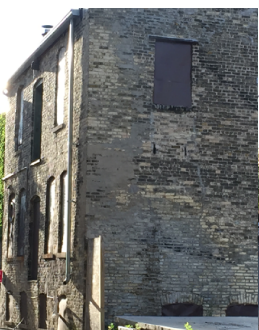
938 W Lapham Blvd. Immediately to the South of 1558. Structural failure.
