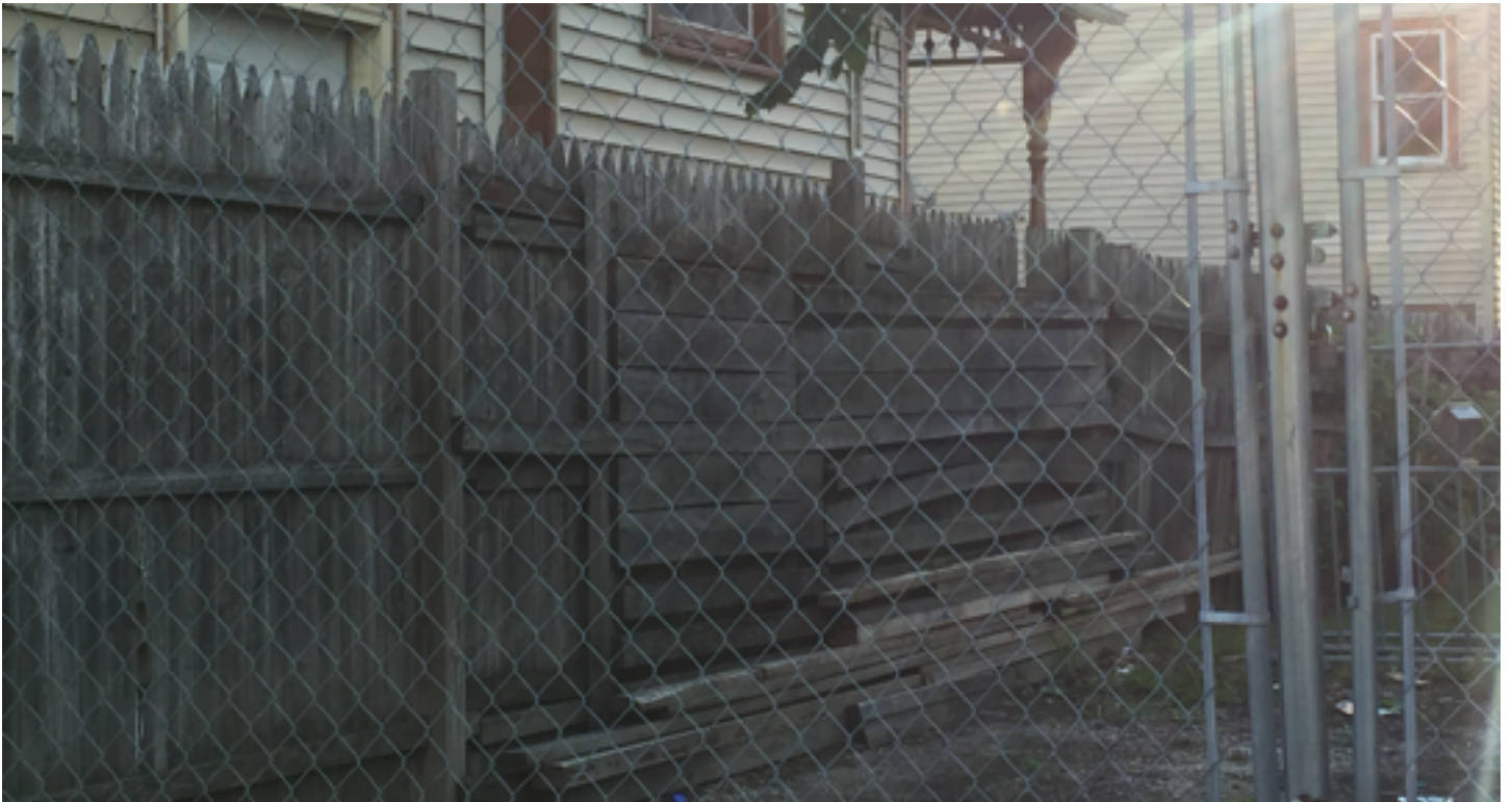
1535? S 10th. Debris/Defective parking area
