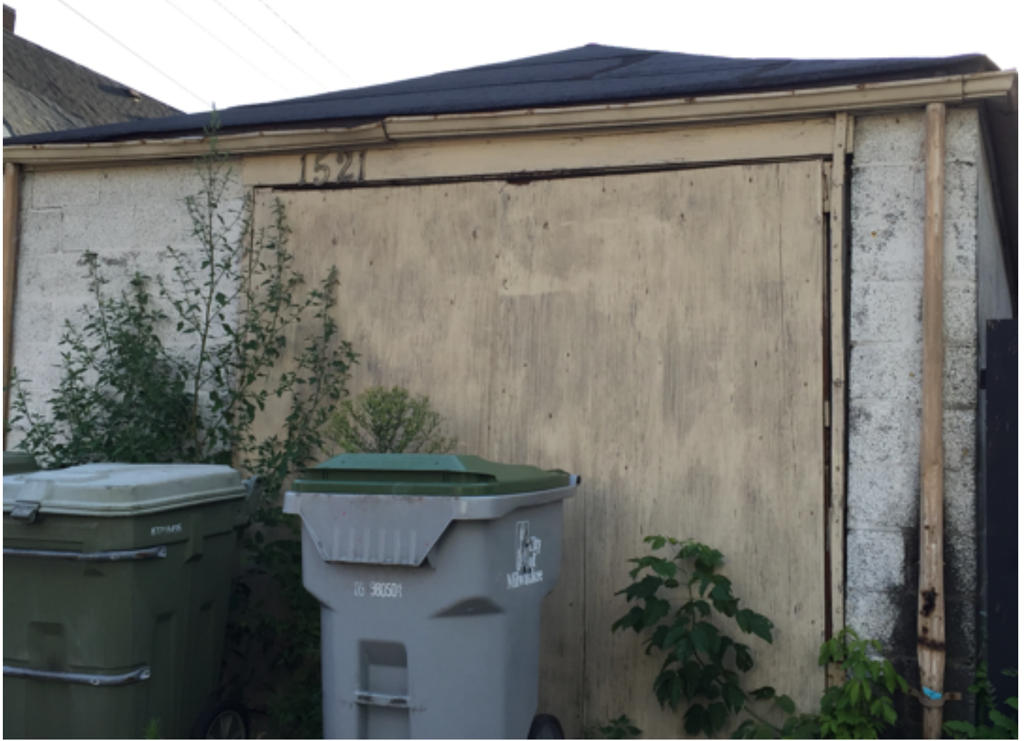
1521 S 10th Defective Garage/Weeds taller than
