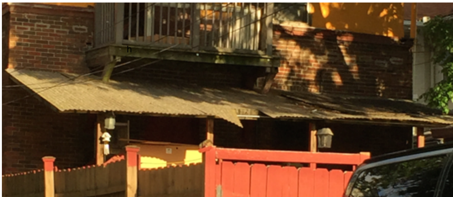
1552 S 10th Two doors north of 1558, across from 1543. Defective roof on rear porch
