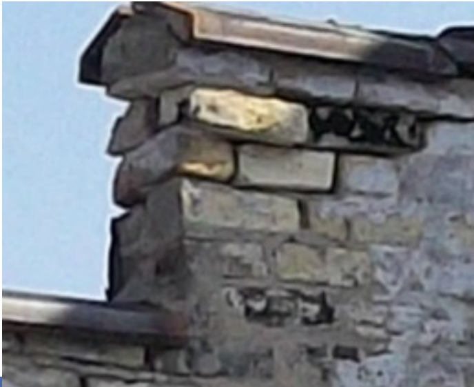
1438 S 6th Adjoining South. Missing windows, failing parapet wall missing siding etc.
