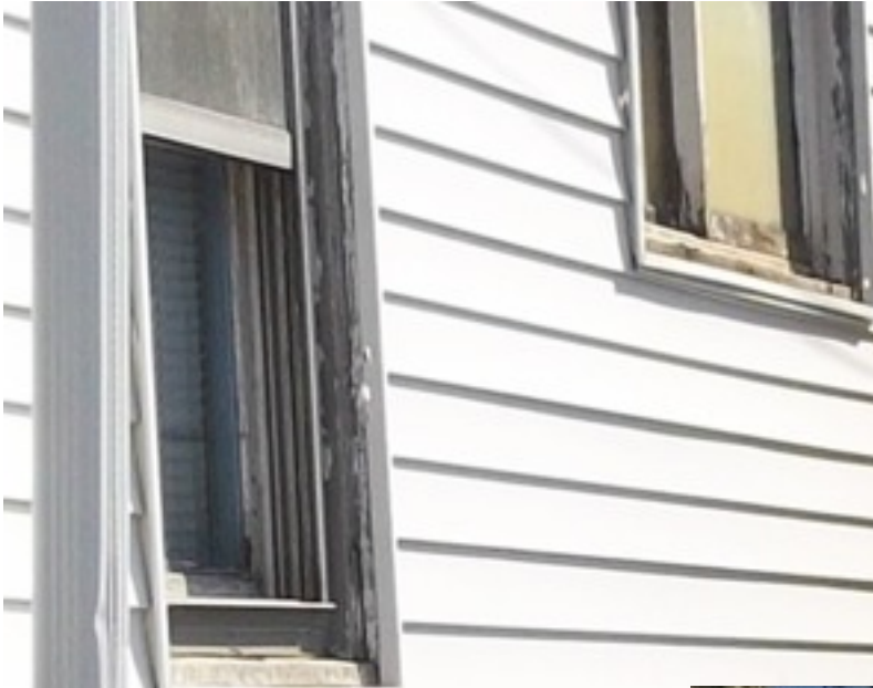
528 W Orchard / 527 W Greenfield Adjoining rear
