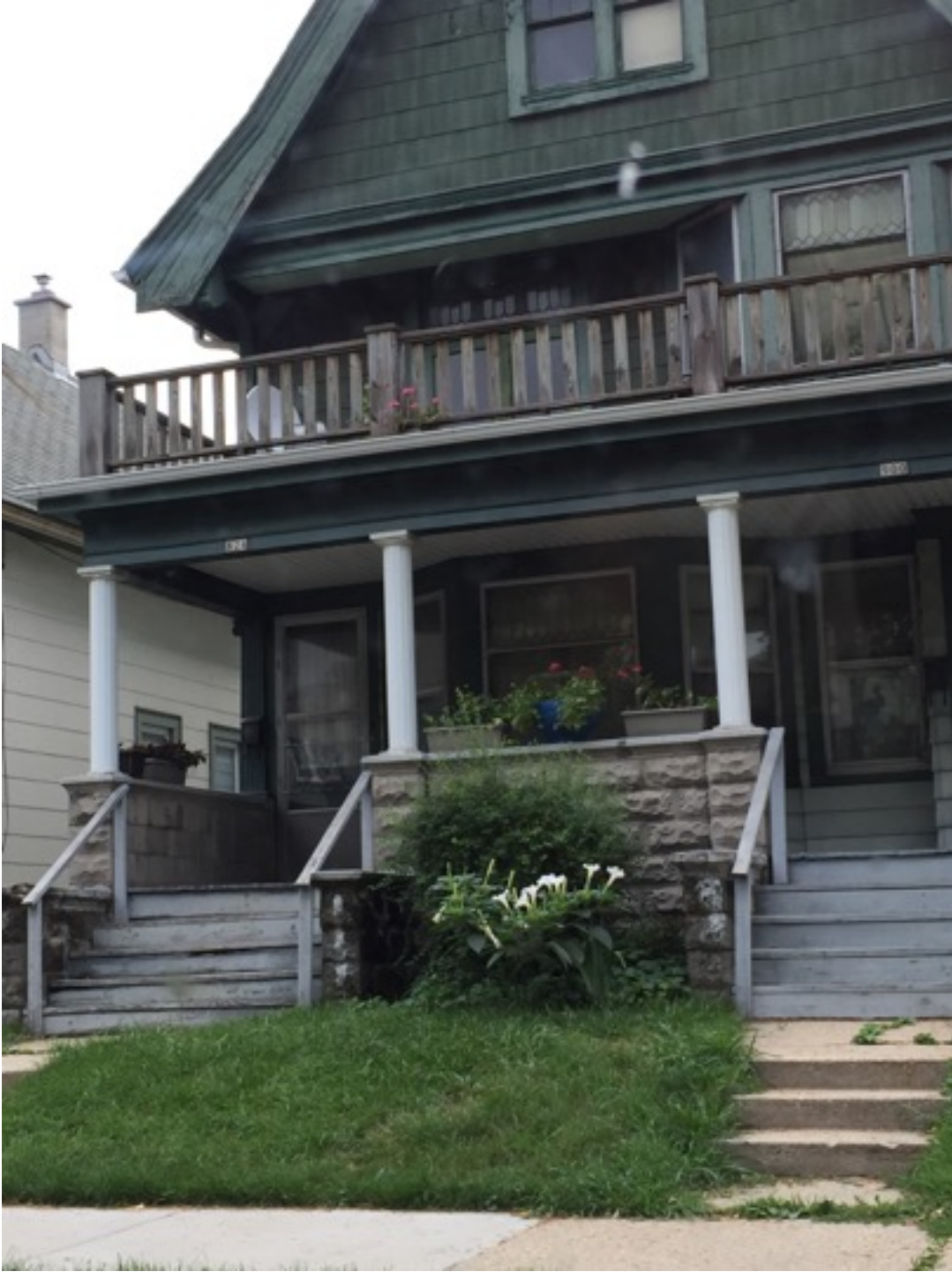
900 S 24th - Paint, Rails, Def Steps
